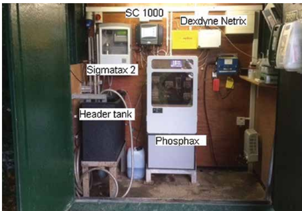
Castledockrell kiosk containing High Resolution Water Quality Instrumentation and telemetry.
