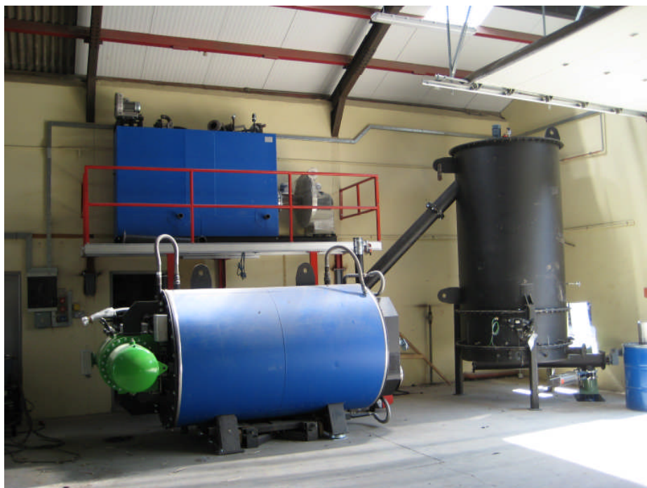
Figure.1. Biomass CHP plant at Oak Park
