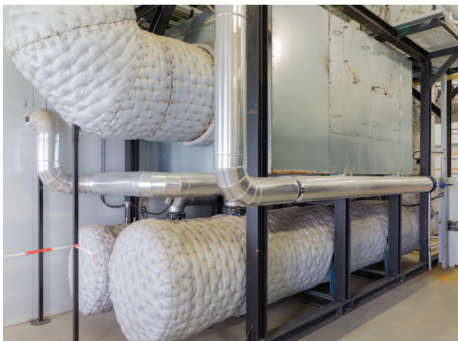
A combined heat and power biomass system.
